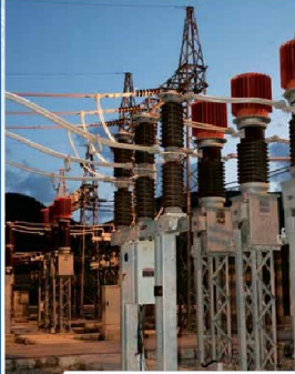
230/63 kV Jirgin (Manasht) Substation
