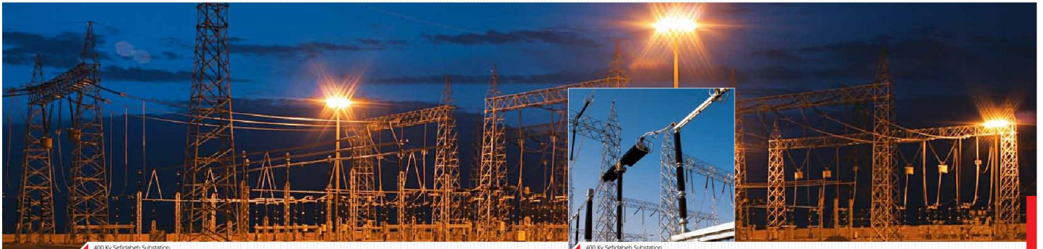
400 Kv Sefidsabeh Substation
