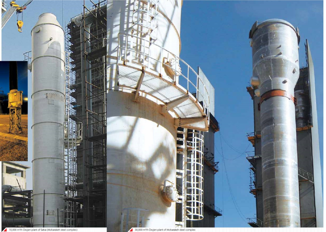
10,000 m 3 /h Oxygen plant of Sabai (Mobarakeh steel complex)
