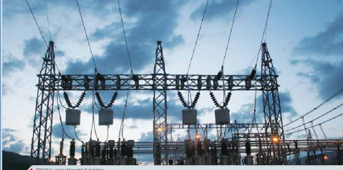
230/63 kv Jarjn (Manesh) Substation
